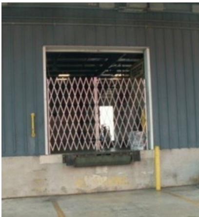
Figure 14 - Scissor Gates are Not Permitted (unless used in combination with additional barrier such as rollup doors)
